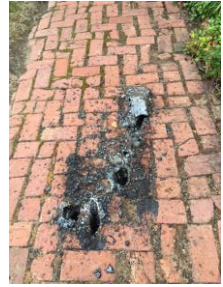
Sidewalk damage at 207 Market St.
